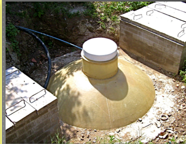
Household biogas digester
