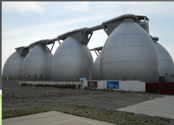
Anaerobic treatment with methane recovery, Bailonggong WWTP, Shanghai
